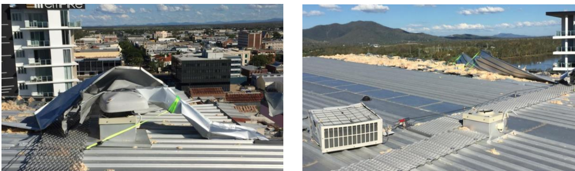
Figure 2. Damage to roof cladding and roof top attachments
