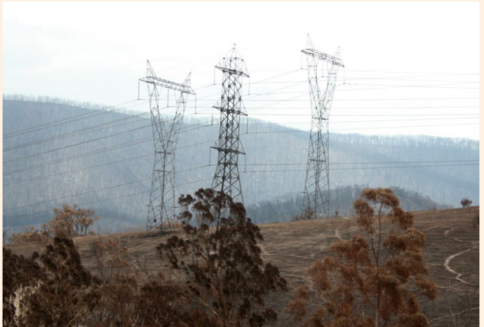
▲ Above: THIS RESEARCH HAS IDENTIFIED THREE DECISION MAKING AREAS ACROSS WHERE RISK OWNERSHIP CAN BE ASSESSED. PHOTO: DAVID BRUCE, BUSHFIRE AND NATURAL HAZARDS CRC.
