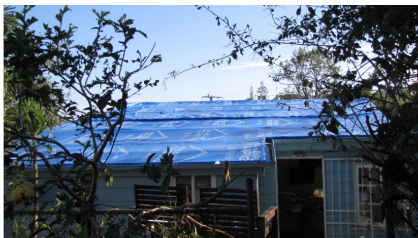
Figure 4: Loss of cladding and battens of an older home. New cladding had been installed onto the original battens.
