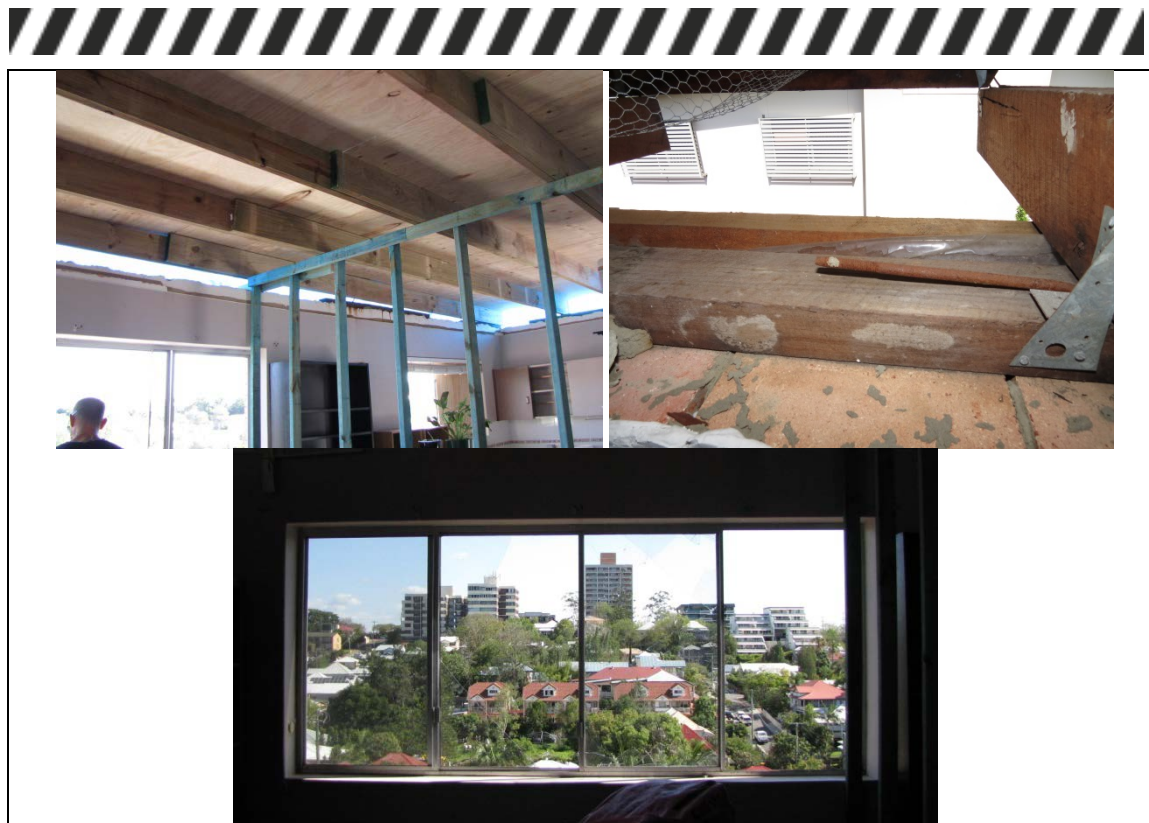
Figure 5: An example of complete roof loss of the top storey unit of a 3-storey apartment building (new roofing currently being installed). Original timber rafters had inadequate tie down to withstand internal pressure due to the breakage of a large southern facing window. The unit was also located on top of an escarpment (outlook shown in the lower photograph) and may have experienced slightly higher wind speeds.
