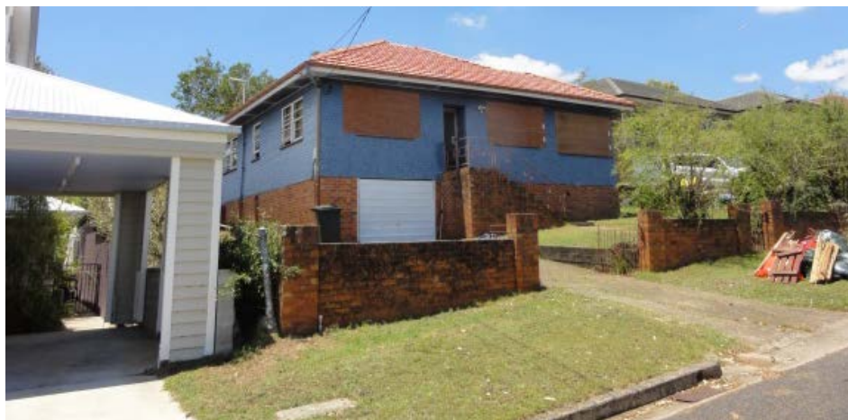
Figure 6: Broken windows on the southern facing wall as well as water damaged goods placed at the front for collection was commonly observed.
