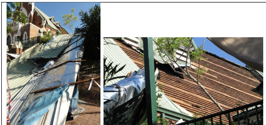
Figure 3: Loss of metal cladding and battens of a church. Originally a tile roof, the new metal roof was only secured to every 6 th timber batten.
