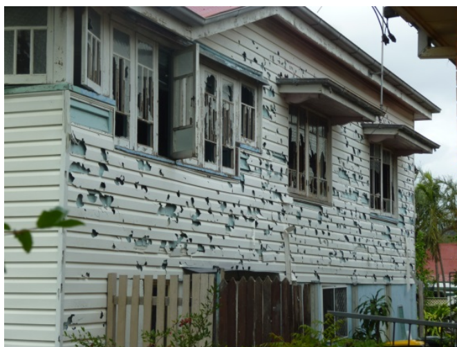
Figure 7: Hail damage to windows and vinyl cladding of an older house. The proximity of the neighbouring house on the right and the size of the window shades suggest hail being driven at a sharp angle by the wind.
