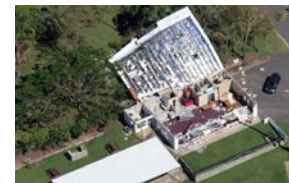
The roof on this clubhouse at a Rockhampton
