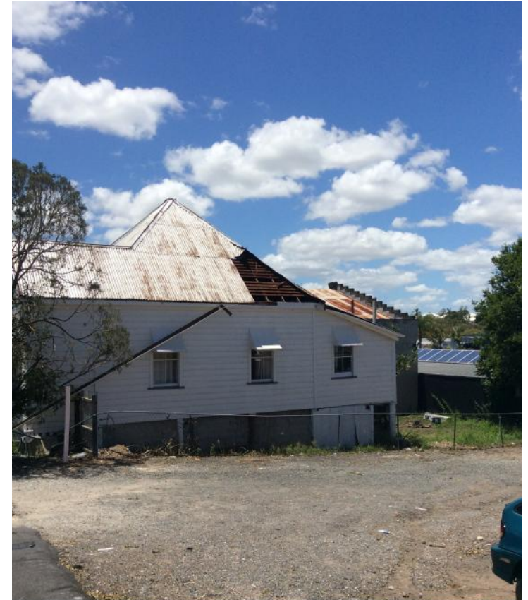
BNE Thunderstorm, partial roof sheeting removed
