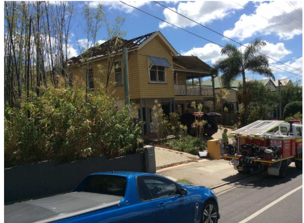
BNE Thunderstorm, all roof sheeting removed
